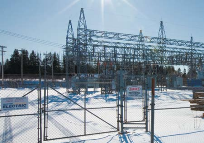
Maritime Electric Substation
