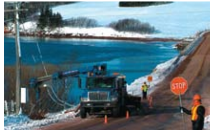
Maritime Electric Line Crew on the scene to remove and replace wires that fell during a storm. Flaggers on site for worker and traffic safety.
